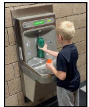
Bottle Filling Station in Winterset public school
